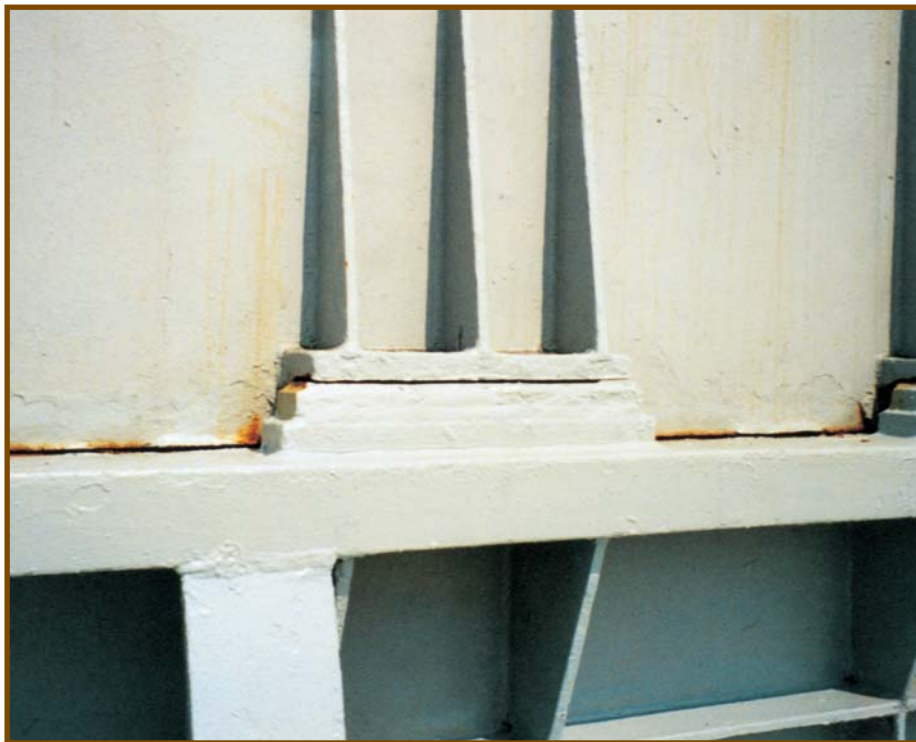
Worn 'steel-to-steel' contact points.
