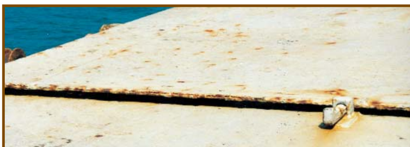
Two panels shown out of alignment.
